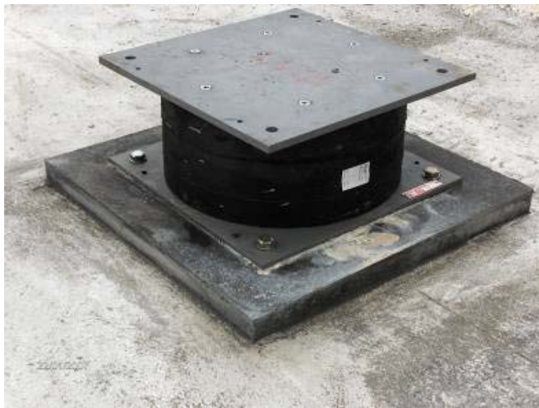
Figure 7 HRDB isolator installed on the foundation
