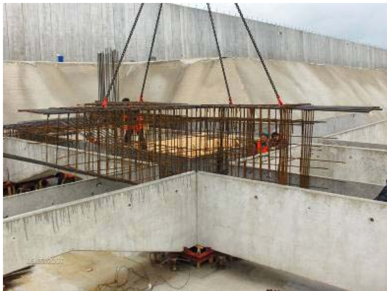
Figure 5 Detail of a beams joint on a rubber isolators; the steel reinforcements are inserted into the precast concrete formwork to obtain the reinforced concrete supporting beam
