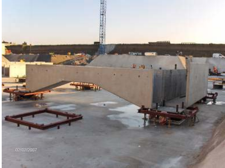
Figure 4 Detail of the building base level laying on the isolation devices, the precast concrete formwork is used to realize the supporting beams to carry the structure and guarantee the suitable stiffness in the horizontal plane. On the left corner the simple steel frame to be placed around the seismic devices is shown
