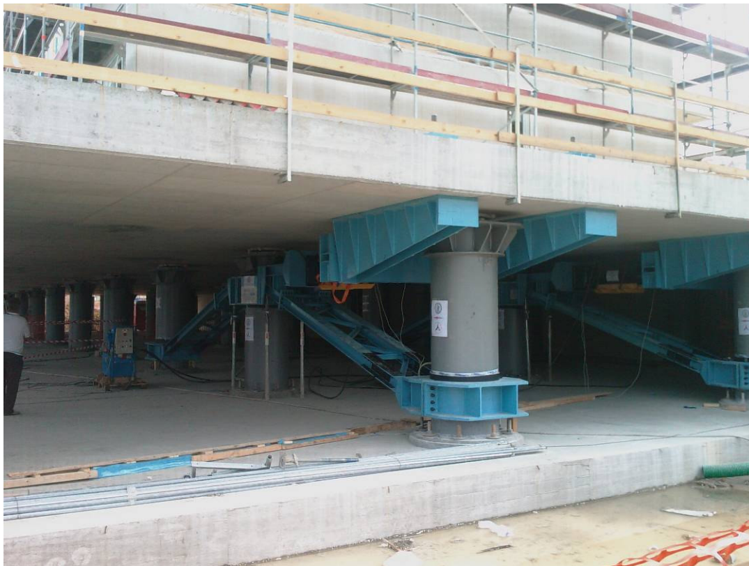
Figure 13 – The reaction frames applied to a building for the execution of the in situ dynamic test
